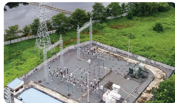
Electricity supply system
