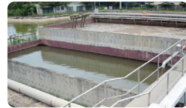
Wastewater treatment system for normal projects • Design capacity: 19,000 m 3 /day.night • Current capacity: 4,000 m 3 /day.night
