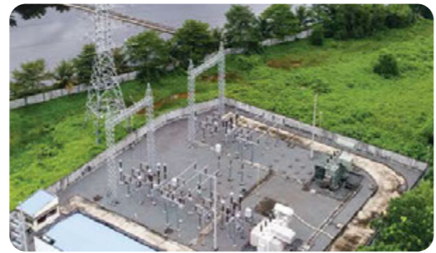
Electricity supply system • Internal station 110KV/22KV • Design capacity 2x63MVA
