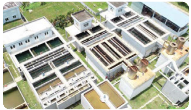
Fresh water supply system • Design capacity: 115,000m 3 /day.night • Current capacity: 20,000m 3 /day.night
